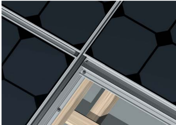
e Installation of the laminates The solar PV laminates fit snugly into the mounting gaskets.
